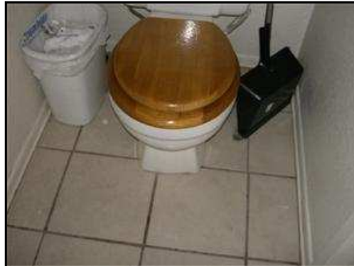
6.7.D Picture 1 Toilet loose at base.
