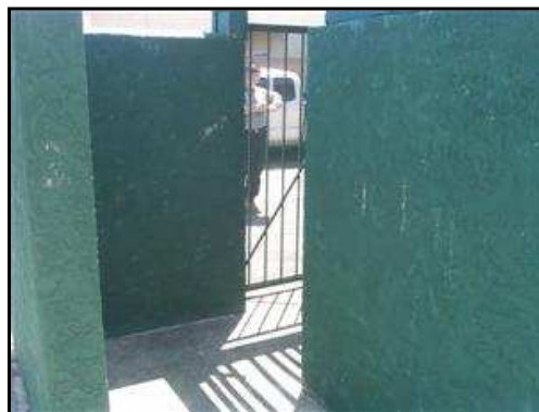
2.8 Picture 4 Trash enclosure missing man door. Recommend consultation with city building department for trash enclosure requirements.
