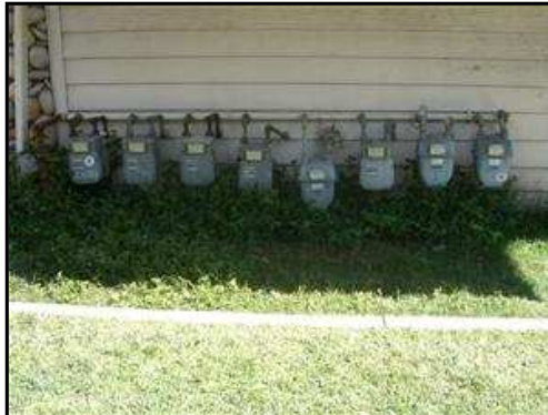
4.5 Picture 1 Gas meters located at back of property.
