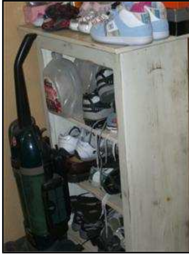
6.21.F Picture 1 Water heater cabinet not accessible.
