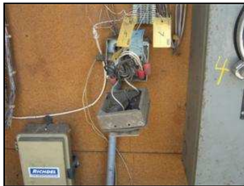
7.1 Picture 2 Quad outlet damaged
