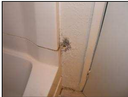
6.1.D Picture 1 Drywall soft with moisture present at time of inspection.
