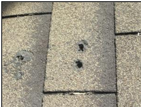
1.0 Picture 1 Penetrations on asphalt shingles.
