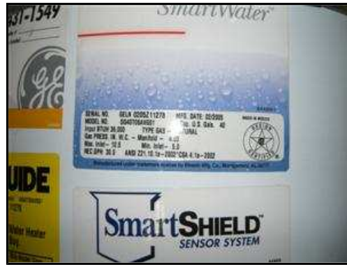
4.2 Picture 10 Water heater nomenclature plate - Unit 5
