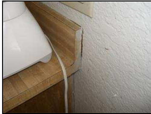
6.5.B Picture 4 Counter top caulking deteriorated.
