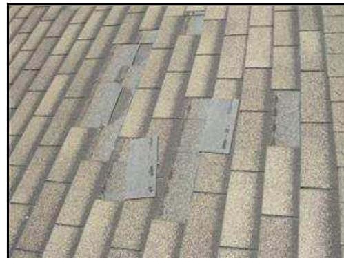
1.0 Picture 2 Asphalt shingles broken.
