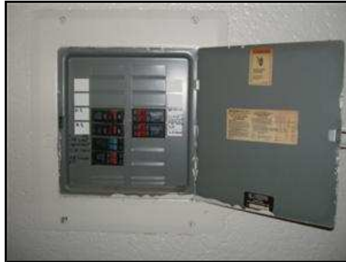
6.23.C Picture 1 Sub panel located behind door in bedroom.
