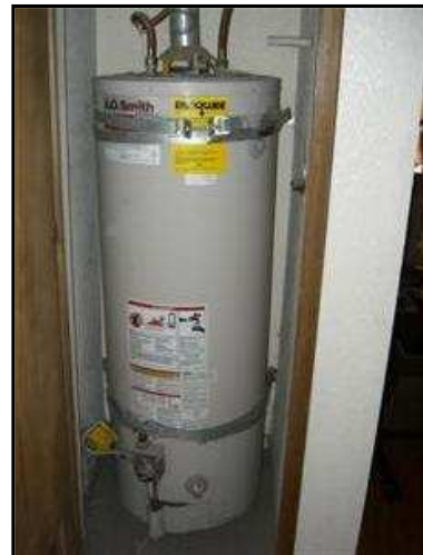
4.2 Picture 8 Water heater - Unit 4
