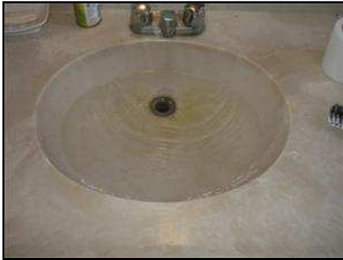
6.5.B Picture 3 Bathroom sink slow drain.
