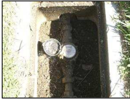
4.1 Picture 1 Water meter located at curb.
