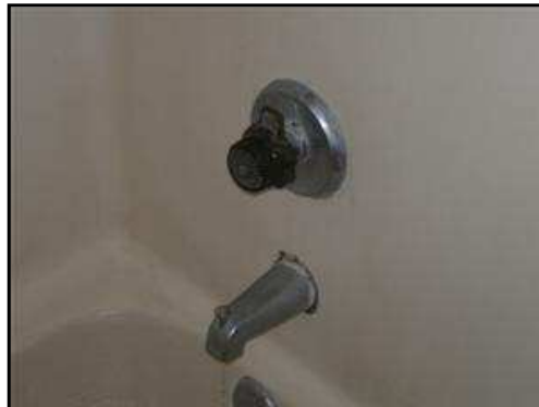
6.6.F Picture 1 Mixing valve damaged.
