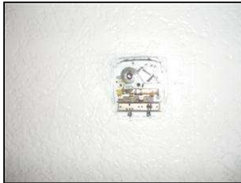
6.18.D Picture 1 A/C & Heating thermostat damaged.
