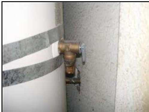
4.2 Picture 7 TPRV drain line disconnected - Unit 1
