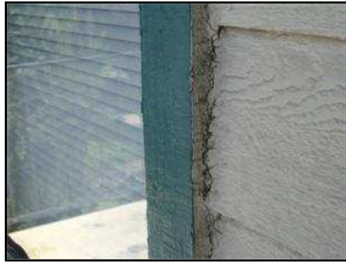
2.0 Picture 4 Caulking deteriorated.
