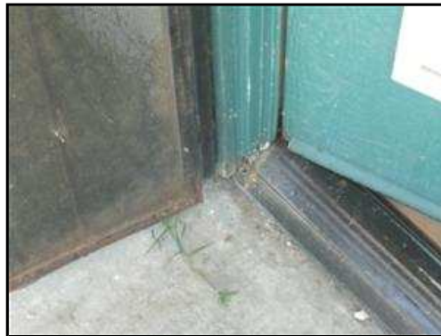
6.3.B Picture 1 Dryrot present at front door jamb - consult termite report.
