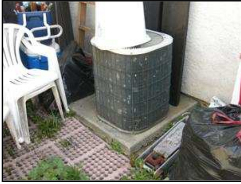
6.16.D Picture 1 Condenser did not respond to signal. Recommend service by qualified technician.
