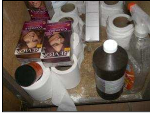
6.5.B Picture 2 Bathroom sink cabinet bottom water damaged - no active leak present at time of inspection.
