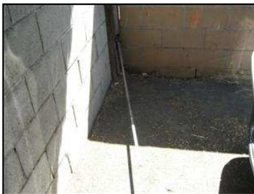
2.0 Picture 1 Trip hazard
