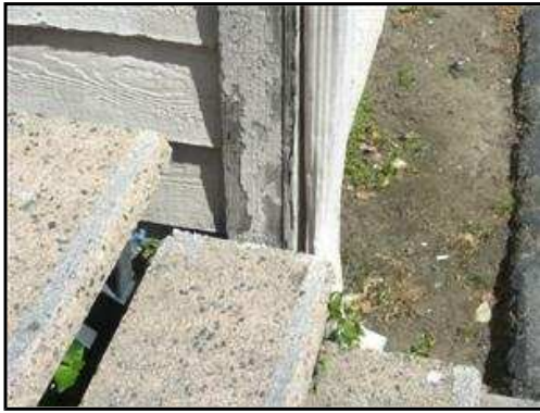
2.0 Picture 3 Dryrot present at wood trim.
