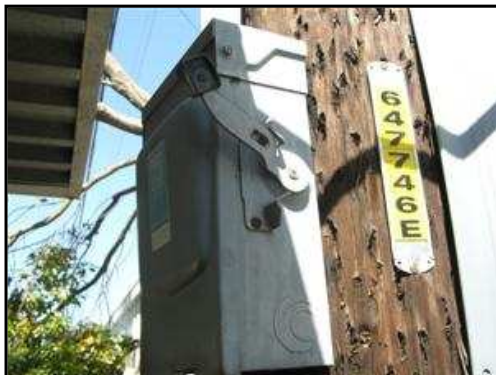
7.0 Picture 1 Pole mounted disconnect
