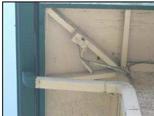
7.0 Picture 2 Improper wiring.
