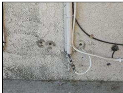
2.0 Picture 2 Excess stucco penetrations.
