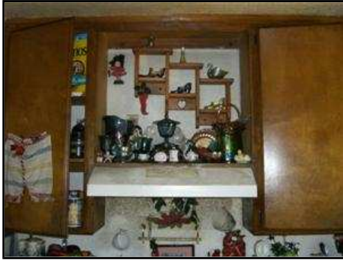
6.11.E Picture 1 Recirculating range hood. cabinet doors missing above range hood.
