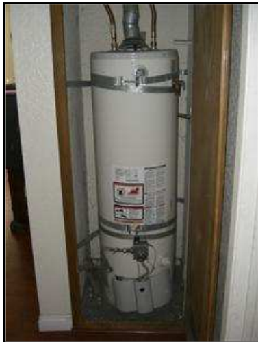
4.2 Picture 5 Water heater - Unit 1
