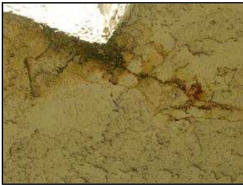
2.3 Picture 1 Rust stains present on underside of front balcony
