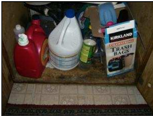
6.5.E Picture 1 Under sink cabinet bottom in kitchen deteriorated. No moisture present at time of inspection.
