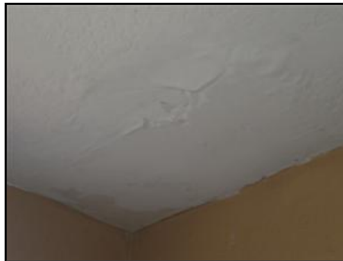
6.0.F Picture 1 Previous ceiling damage in bathroom above tub.
