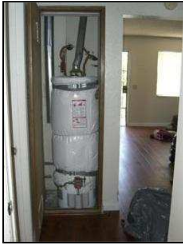
4.2 Picture 3 Water heater - Unit 3
