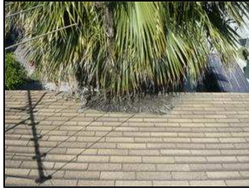
1.0 Picture 3 Palm tree in contact with roof asphalt shingles.
