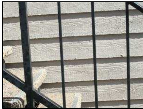
2.3 Picture 2 Stair railing spacing greater than 4"
