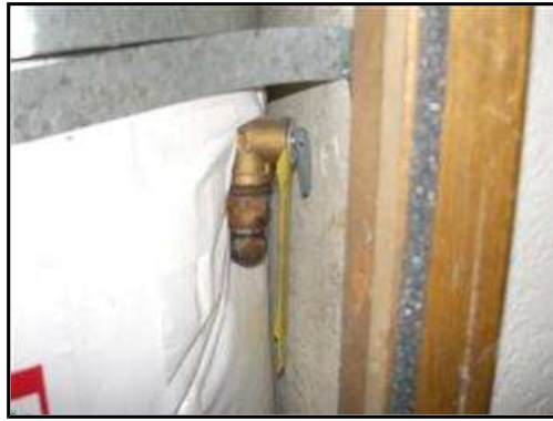
4.2 Picture 4 TPRV drain line disconnected.
