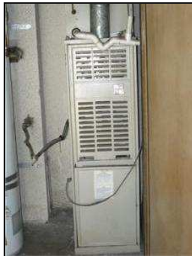
6.14.D Picture 1 FAU located in cabinet - kitchen area.
