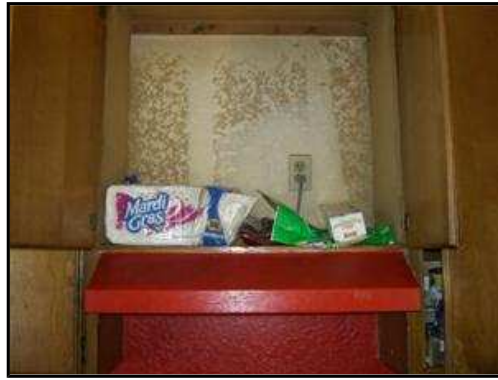
6.11.B Picture 1 Re-circulating range hood typical all units
