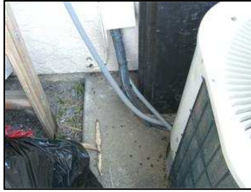
6.16.D Picture 2 Refrigerant line insulation serviceable.
