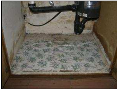
6.5.A Picture 1 Evidence of previous water leak under kitchen sink.
