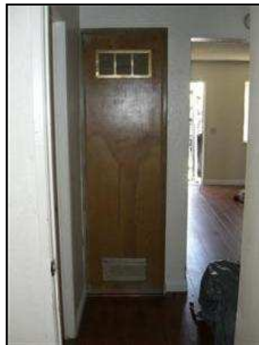
4.2 Picture 2 Water heater closet - Unit 3
