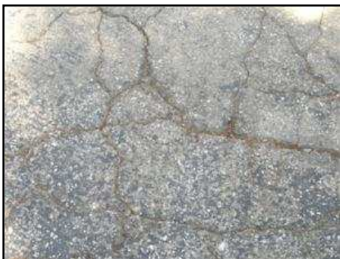
2.8 Picture 3 Alligating present at asphalt driveway.
