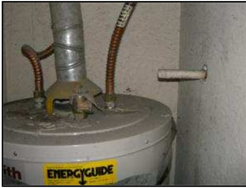
4.2 Picture 9 TPRV disconnected - Unit 4
