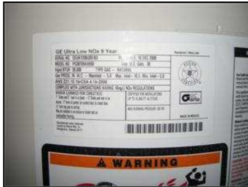
4.2 Picture 6 Water heater nomenclature plate - Unit 1
