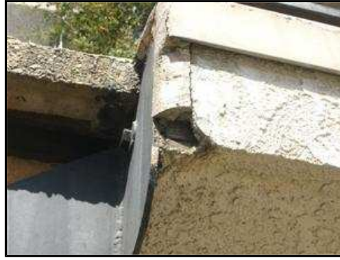
2.3 Picture 6 Minor stucco damage to balcony corner.
