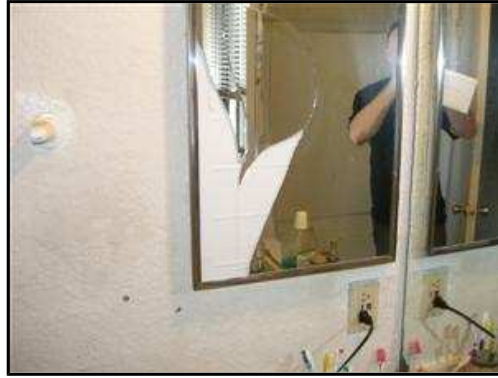
6.5.D Picture 1 Medicine cabinet mirror broken.
