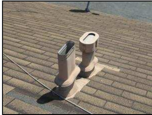
1.3 Picture 1 Vent cap missing.
