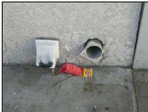
4.2 Picture 1 Dryer vent damaged.
