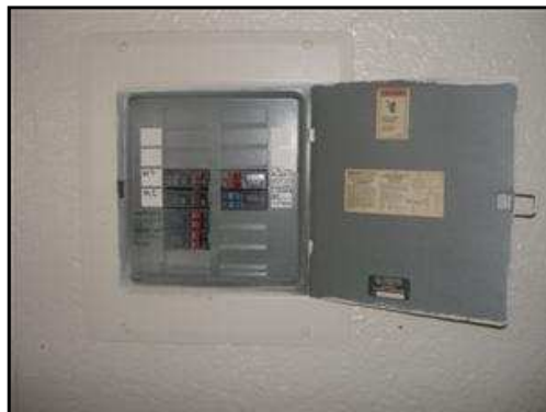
6.24.B Picture 1 Sub panel located behind
