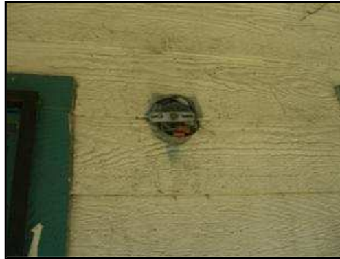
6.26.B Picture 1 Porch light fixture missing.
