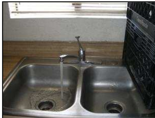
6.6.A Picture 1 Faucet loose. recommend repair.
